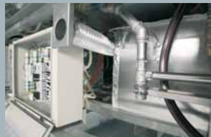
Installation for energy and water supply
